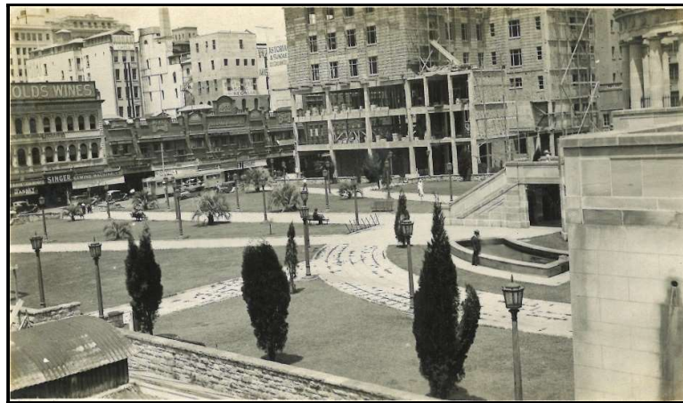
Anzac Square and first stage of state government buildings under construction, ca 1932 (Courtesy Ean & Rachael Rice)
